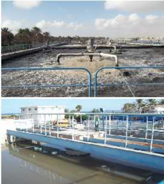
Pictures illustrating aeration units at the existing Gabès WWTP
